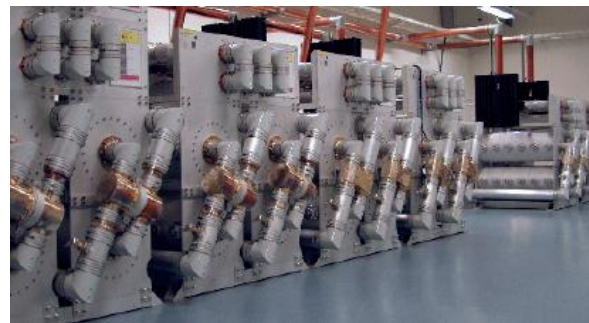
Figure 12. A typical digital/analogue combiner chain in Sweden(Exir Broadcasting and Telecom) (The first analogue combiner is a patch panel. To the left is space reserved for the forthcoming extension of channels 5 and 6)
